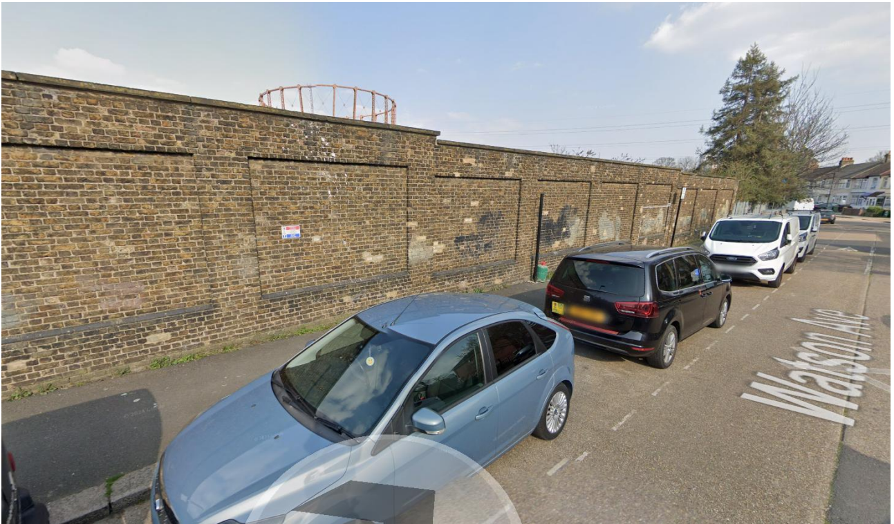
Figure 3 – Photograph taken from south-west of the site showing the retained boundary wall with the gasholder partly visible.
