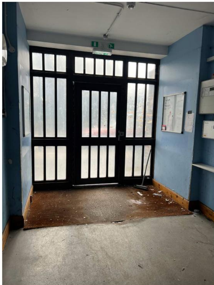
Existing door treatment impedes visual connection between street and reception
