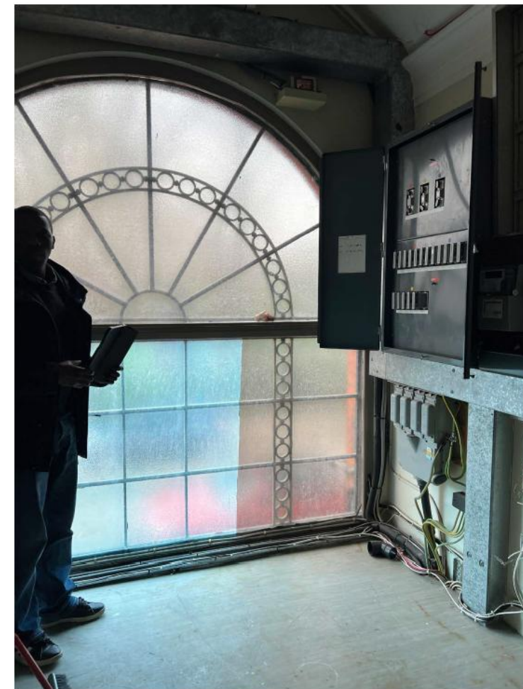
Space above the main entrance seen with electrical services unit
