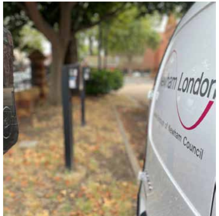
EV charger at East Ham Town Hall
